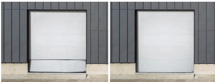
DAMAGED COMPETITIVE DOOR
